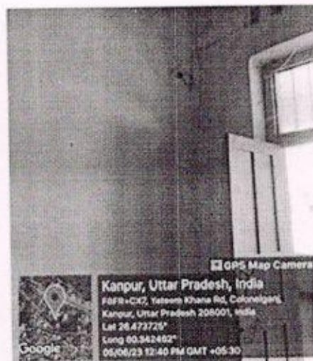
CCTV Camera, Room No. 25
