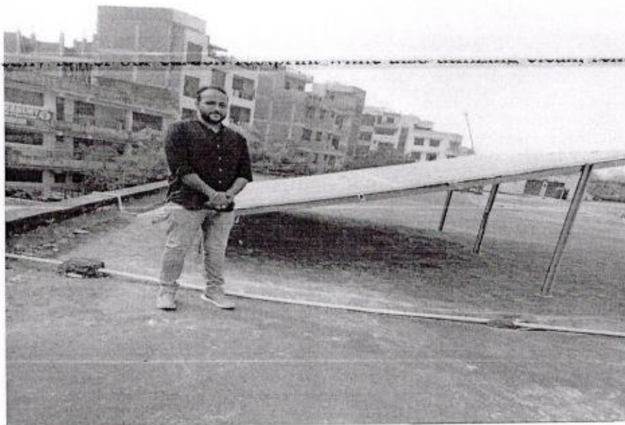
Solar Panel installed on roof top
