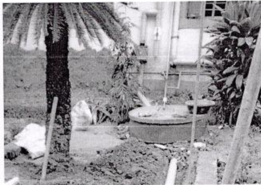
Rainwater conservation pit in botanical garden of college
